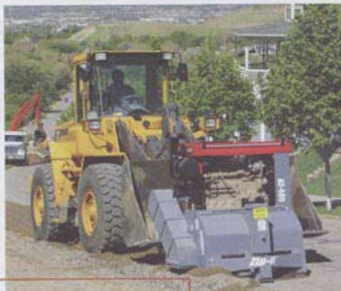
A Utah contractor finds the AZ480 can grind a 1,000-foot trench 48 inches wide through 6-inch asphalt in about an hour.
