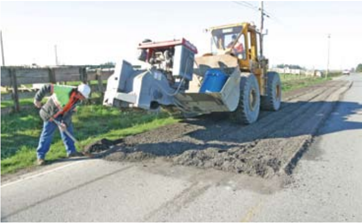
Asphalt Zipper model AZ-360 shown recycling in-place, a 200 x12 foot patch. The site was recycled and ready for paving in less than 2 hours.
