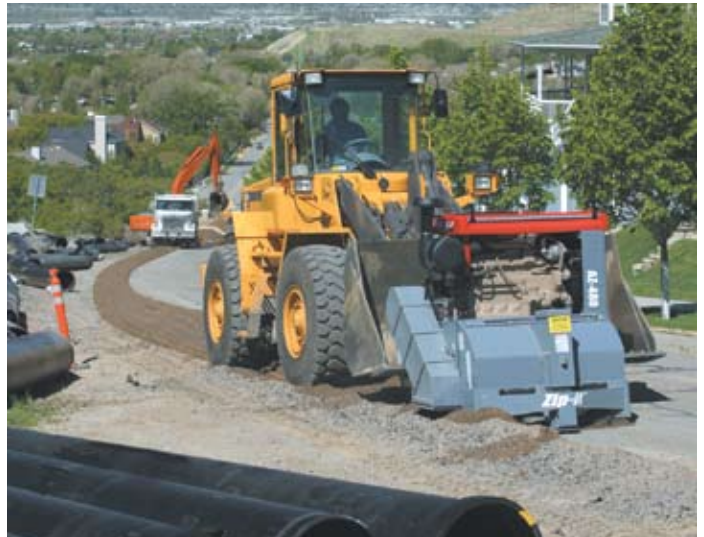
The Asphalt Zipper can open more trench in 30 minutes than most crews can lay pipe in an eight hour day. Many construction companies use one Zipper to service multiple crews because of its speed and portability.
